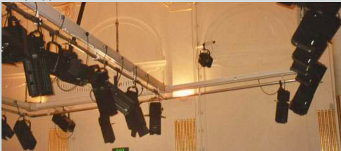
New lighting grid.
